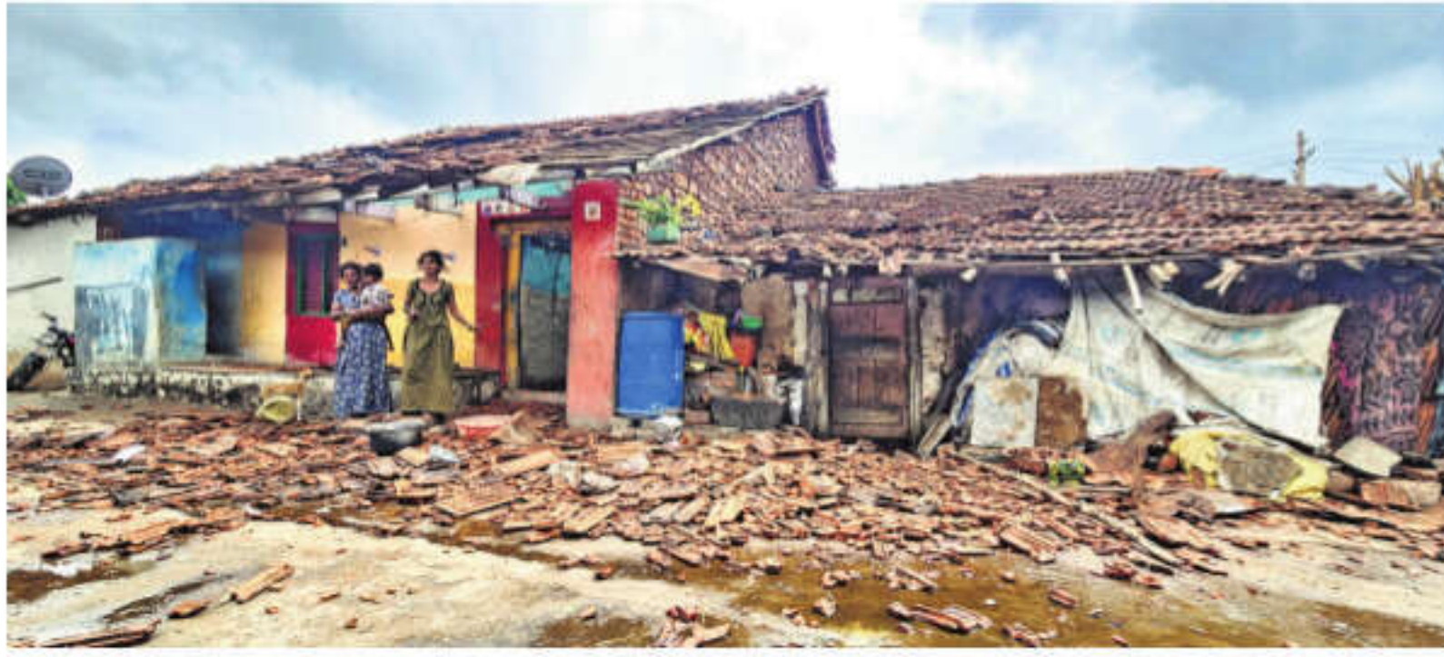
A view of the vandalised house of Yallappa in Bharamyanatti village in Belagavi taluk | EXPRESS
