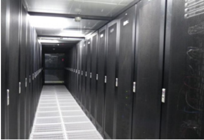
RailTel Data Center at Gurugram
