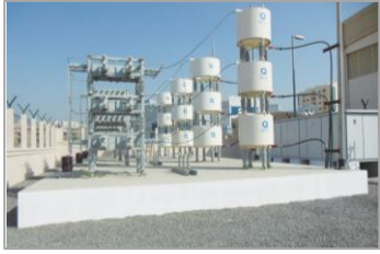
Capacitor Banks Upto 245kV
