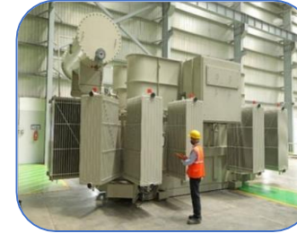
Oil filled reactors
