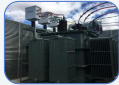
Magnetically controlled reactors
