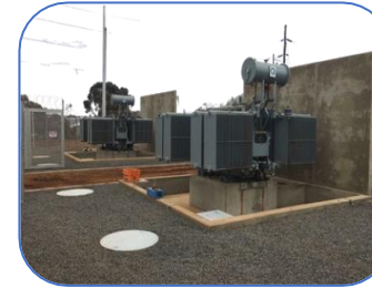
Converter duty transformers
