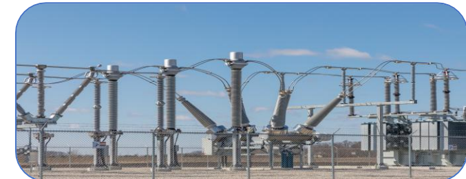
Capacitive voltage transformers and discharge coils
