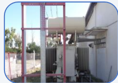
Thyristor controlled reactors
