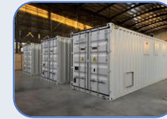
Battery energy storage systems
