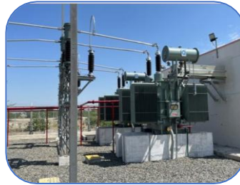
Special purpose transformers
