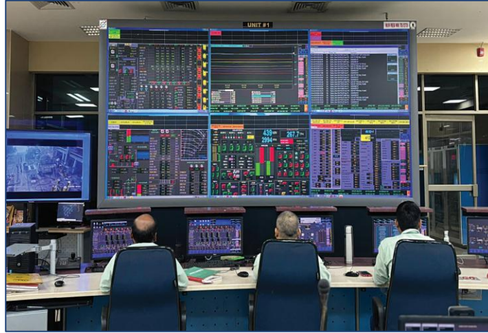
Comprehensive O&M of 2 X 600 MW Singareni STPP, Telangana
