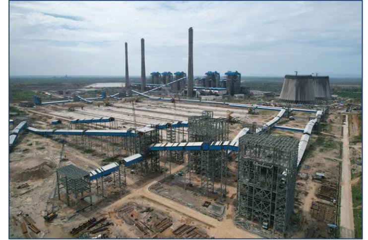
5 X 800 MW Yadadri Thermal Power Station, Telangana
