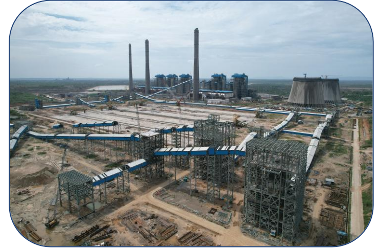
5 X 800 MW Yadadri Thermal Power Station, Telangana
