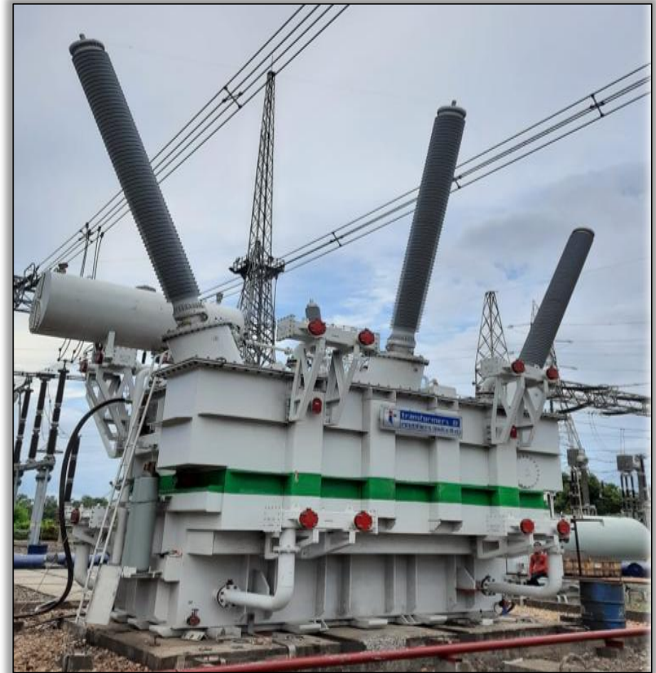
315 MVA, 400/220 kV at HVDC Bhiwadi substation
