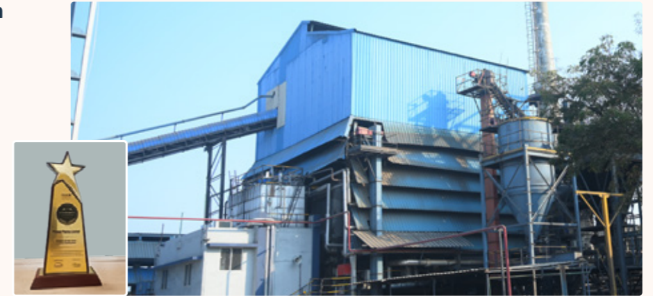
Biomass boiler at Digwal, India
