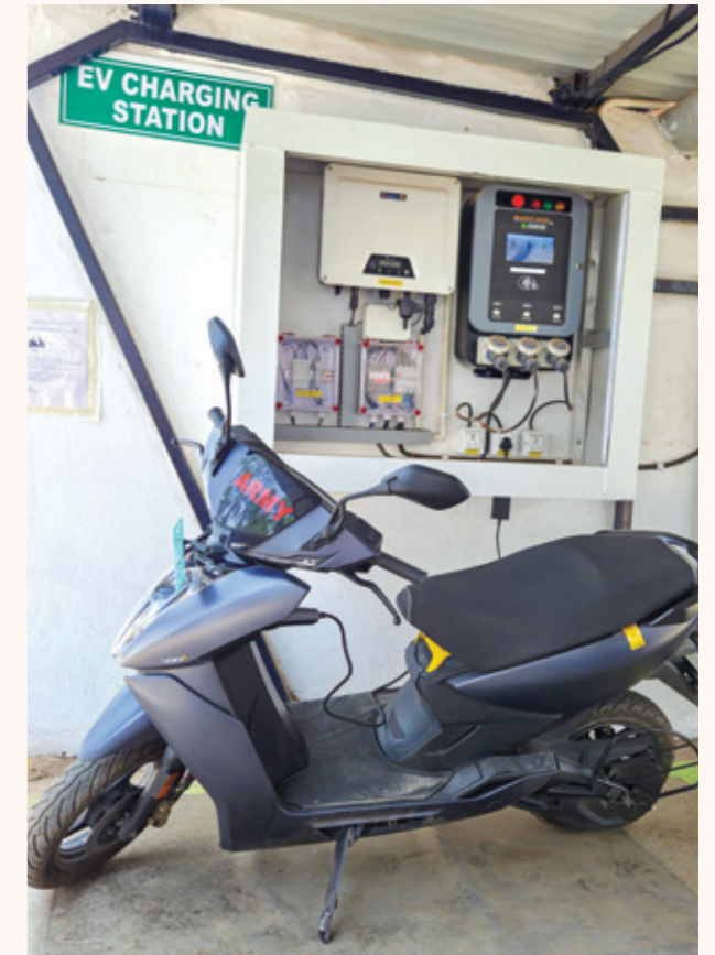
Electric Vehicle Charging Station at Pithampur, India
