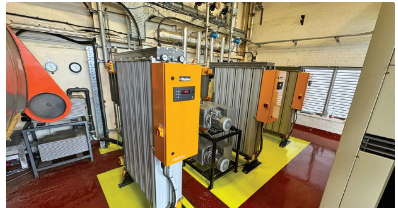
New compressed air dryer at Morpeth, UK
