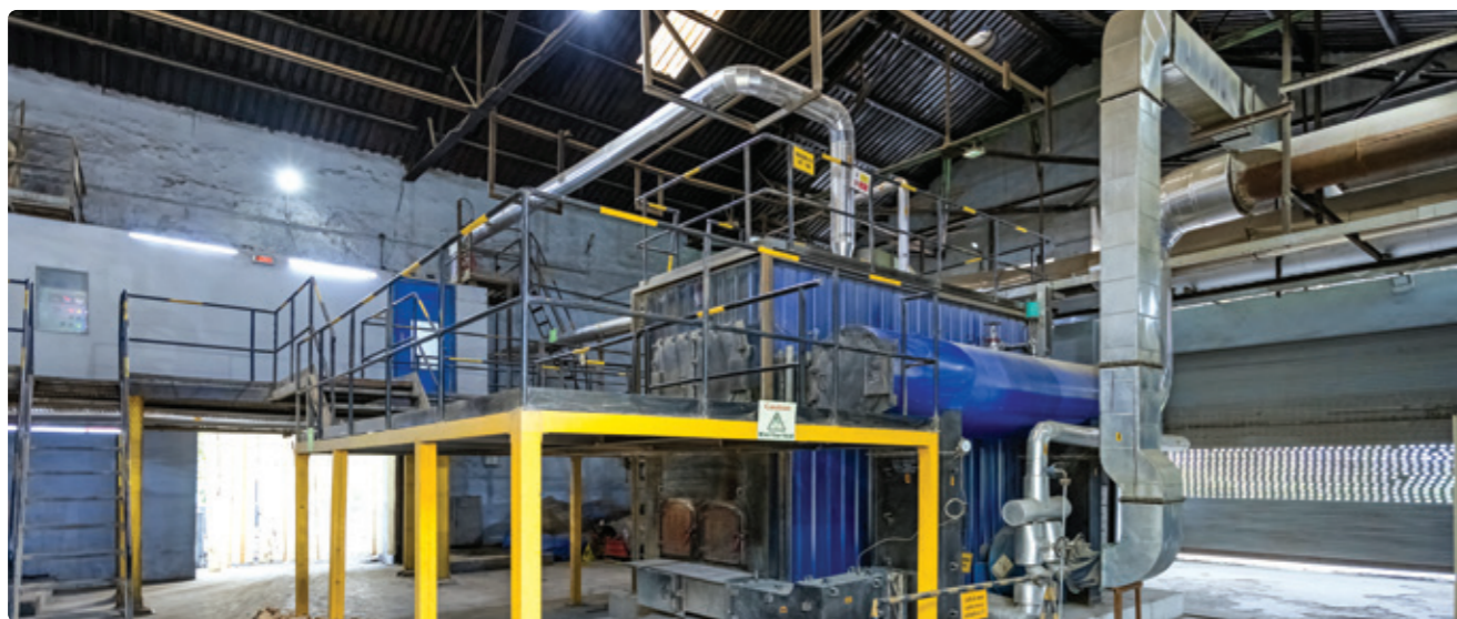
Biomass boiler, Pithampur, India
