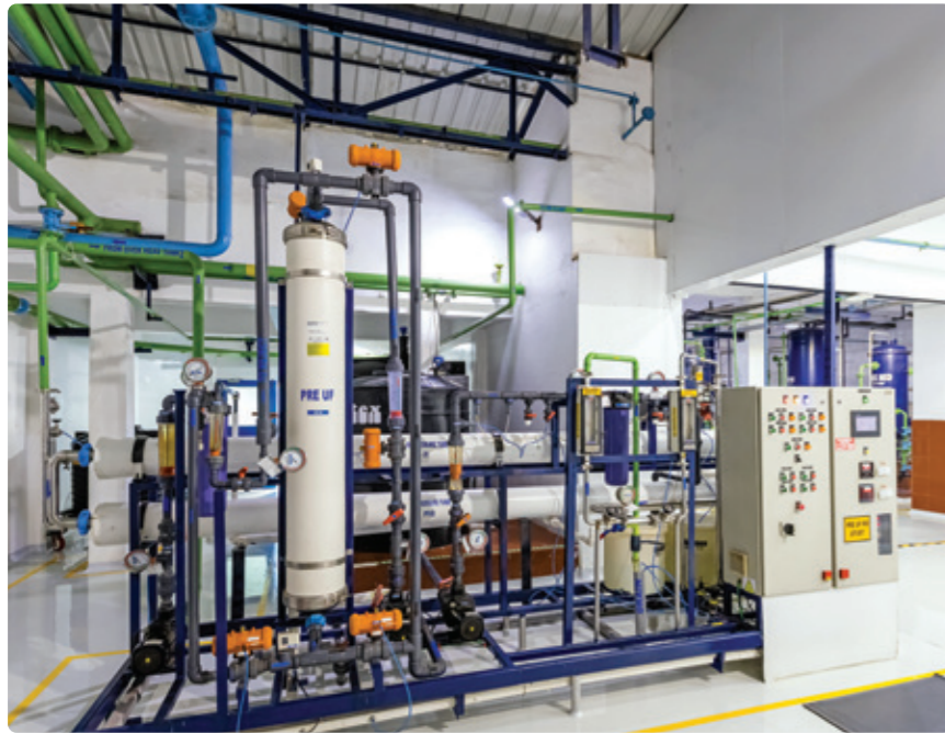
Water treatment plant at Pithampur, India
