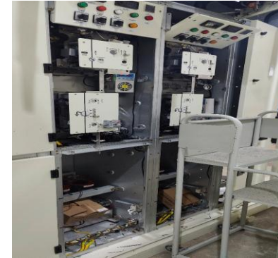
Gas Insulated Switchgears (GIS)
