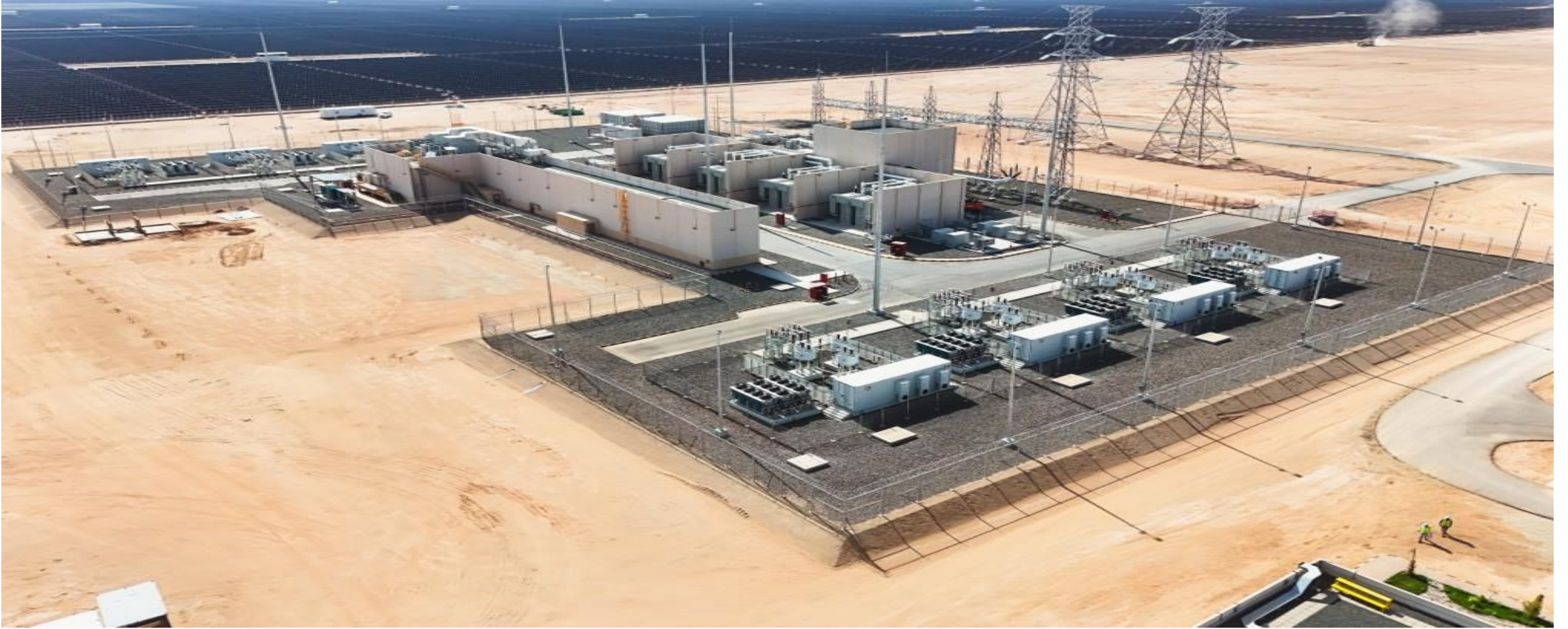
Al Muwayh, Solar PV Project in Saudi Arabia
