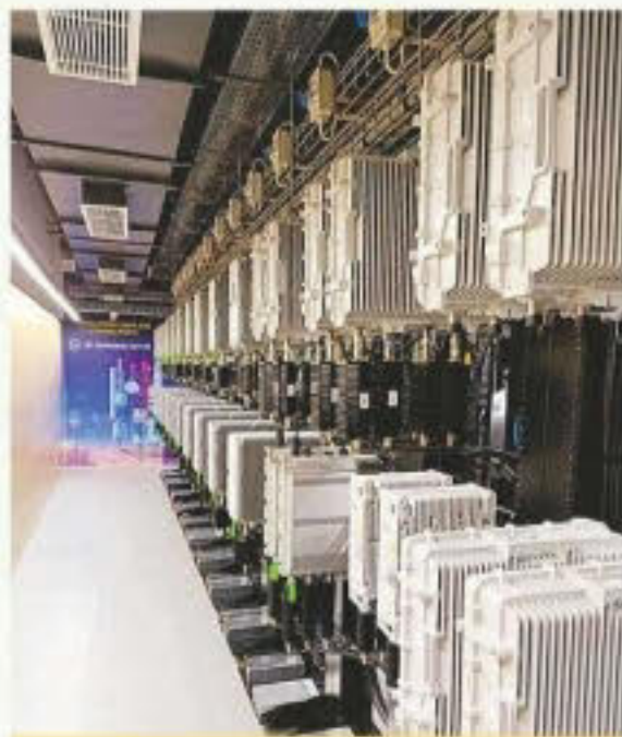
5G Centre to Power Tomorrow's Services
