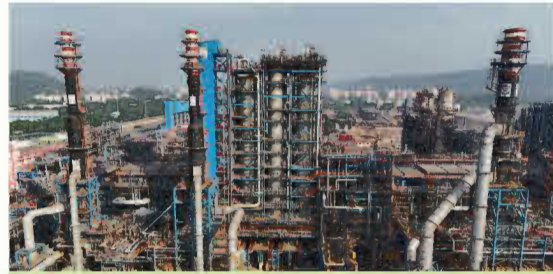
Residue Upgradation Facility (RUF), HPCL Vizag Refinery, Andhra Pradesh
