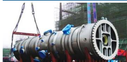
Coal Gasifier for China
