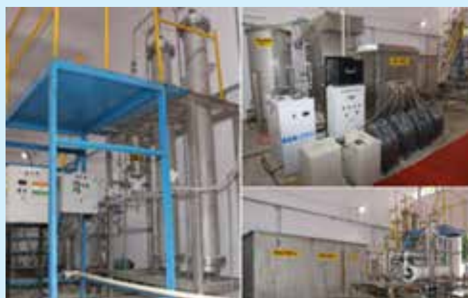
AEWTP installed at North Santhal, Mehsana Asset
