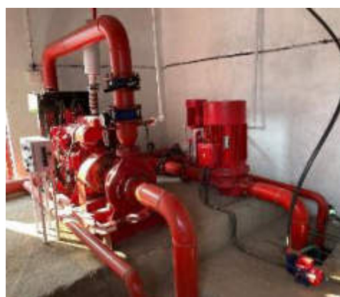
Operational fire pump room
