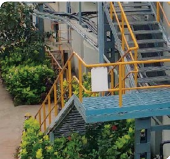
^ ETP-ZLD system at Mekaguda
