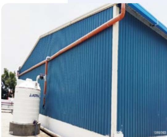
Rainwater harvesting facility at Kothur unit
