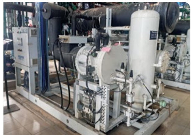
Energy efficient chillers
