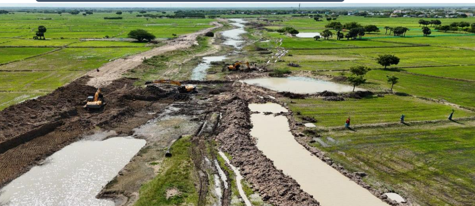
Building irrigation tanks - Expected to enhance water retention in the semi-arid region, supporting agriculture post-monsoon while promoting water conservation and
