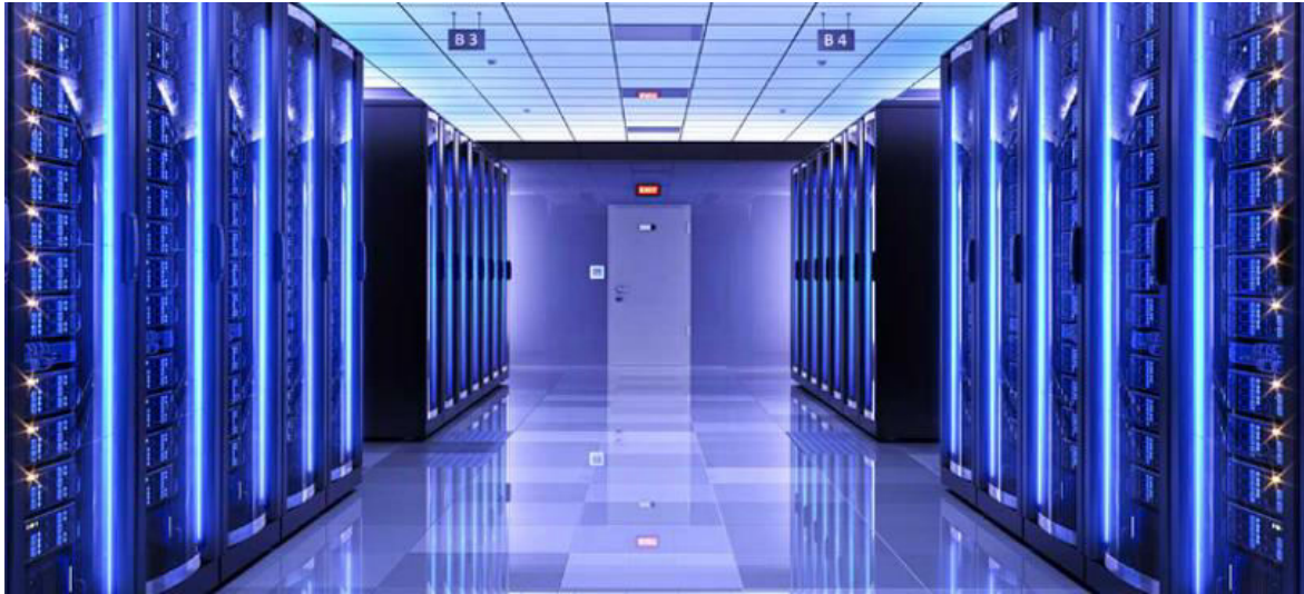
Data Centre Infrastructure Solutions
