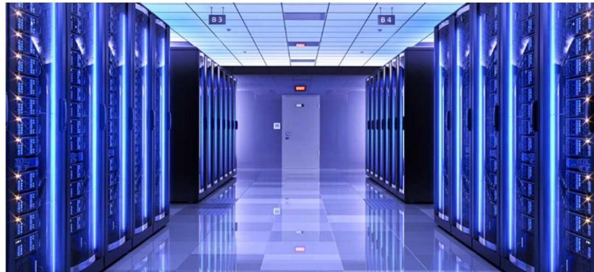
Data Centre Infrastructure Solutions
