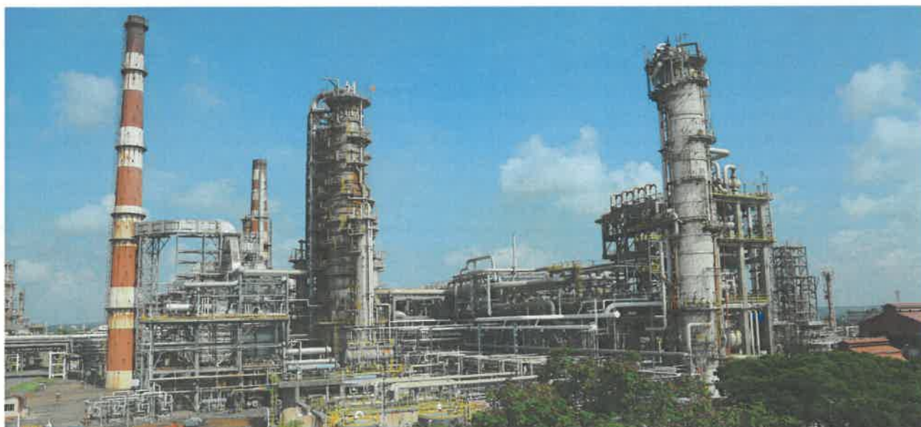
Crude Distillation Unit
