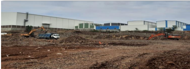
Minda Instrument Cluster Plant Pune
