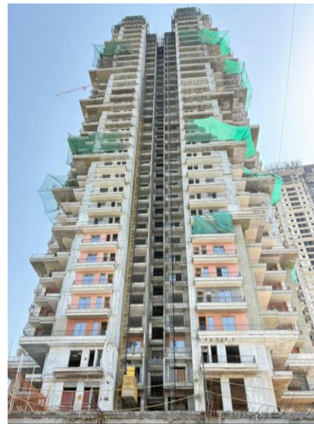
Tower 1 – As on 30 th April 2026 – Thirty fifth floor slab is being casted.
