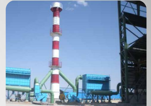
Fume Extraction System
