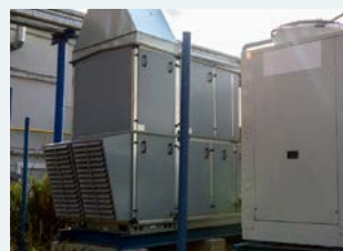
Air Handling Units
