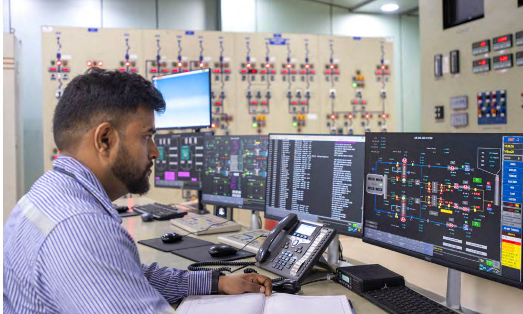
JSW Energy Vijayanagar Power Plant
