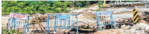
Traffic barricades placed near the damaged Dudhija bridge after heavy rain washed away a section of the bridge at Dudhija on the outskirts of Siliguri, West Bengal
