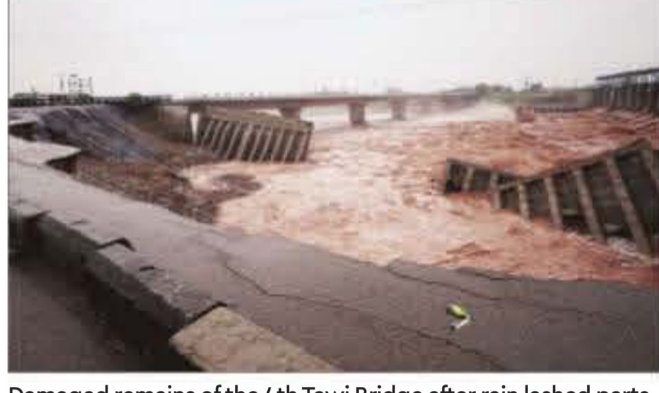
Damaged remains of the 4th Tawi Bridge after rain lashed parts of the city in Jammu on Wednesday
