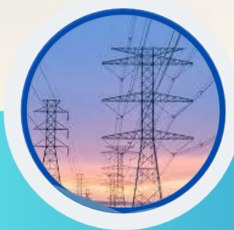
Overhead Transmission Lines
