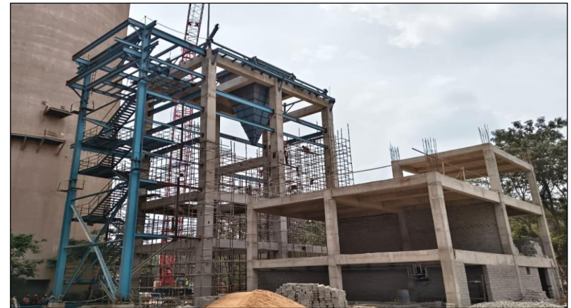
Nandyal IU: Chlorine Bypass - Baghouse and MCC Room
