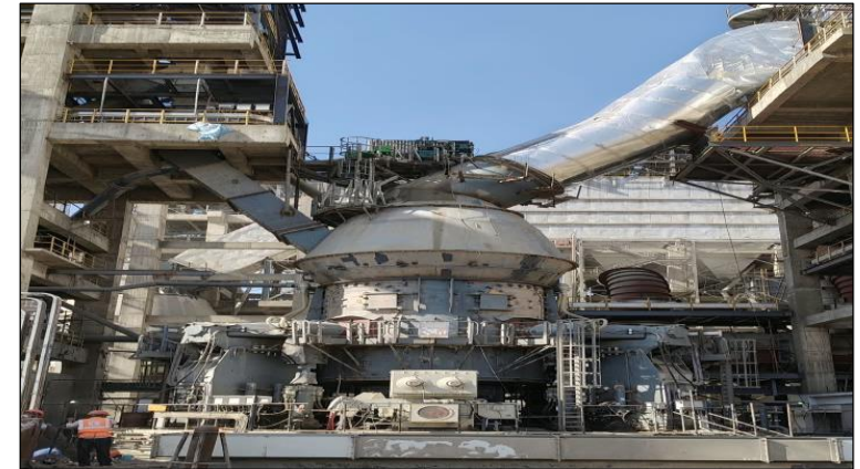
Nagaur 1 MTPA – Cement Grinding Mill
