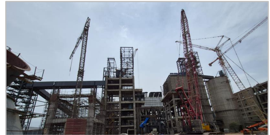
Nagaur IU – Cement Grinding and Packing & Dispatch
