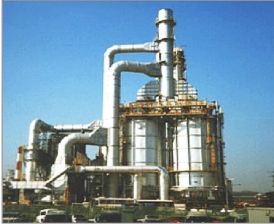
Process Fired Heaters
