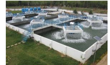
Slow speed fixed aerator
