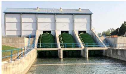
Hydropower Screw Generator
