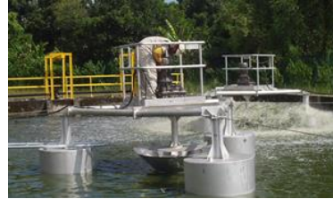
Slow speed floating aerator
