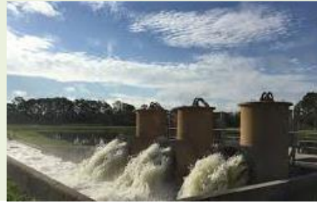
Storm water pumping stations
