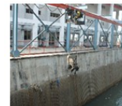
Suspended Trash Rack
