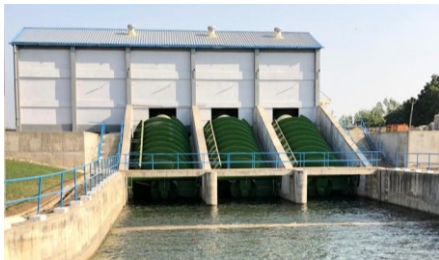
Hydropower Screw Generator
