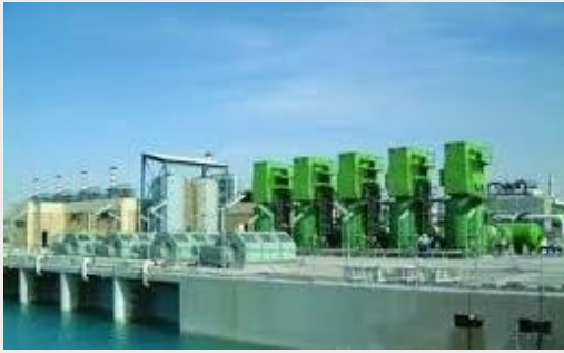
Water intake systems
