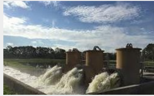
Storm water pumping stations
