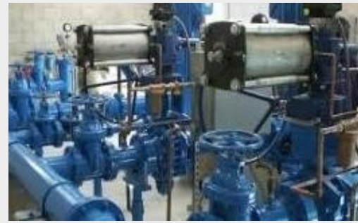
Water & waste water treatment plants
