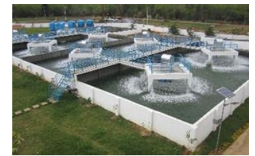
Slow speed fixed aerator
