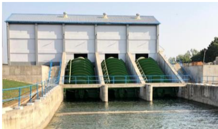
Hydropower Screw Generator
