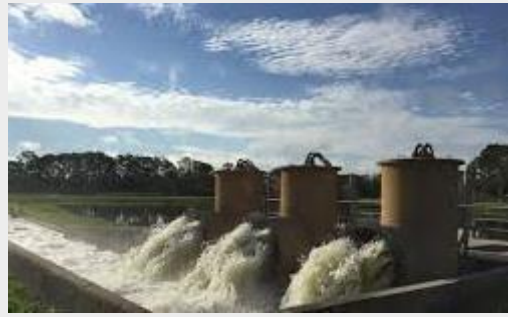
Storm water pumping stations
