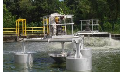
Slow speed floating aerator
