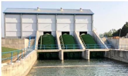
Hydropower Screw Generator
