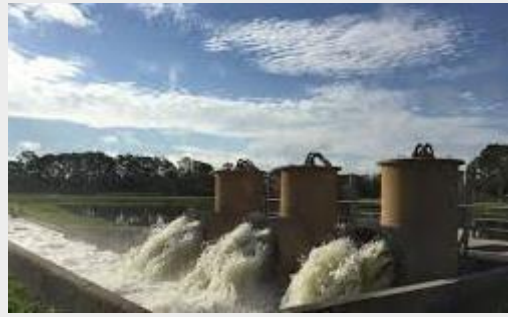
Storm water pumping stations
