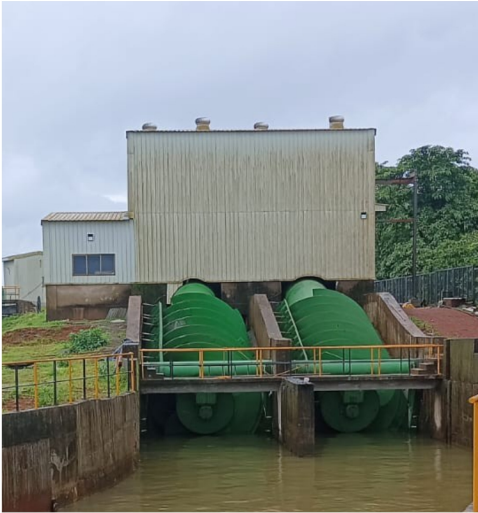
2 X 235 kW Archimedean Screw Turbine
