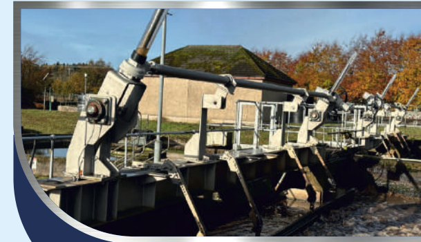
Shotts Waste Water Treatment Works, Glasgow, UK
