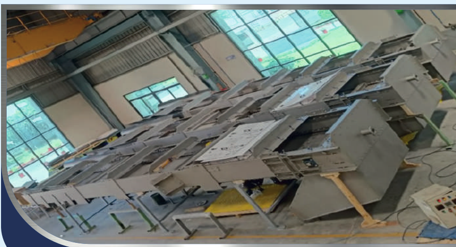
200MLD Al Haer, Independent Sewage Treatment Plant, KSA
