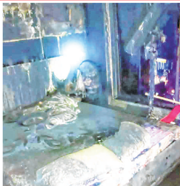
One of the gutted flats
