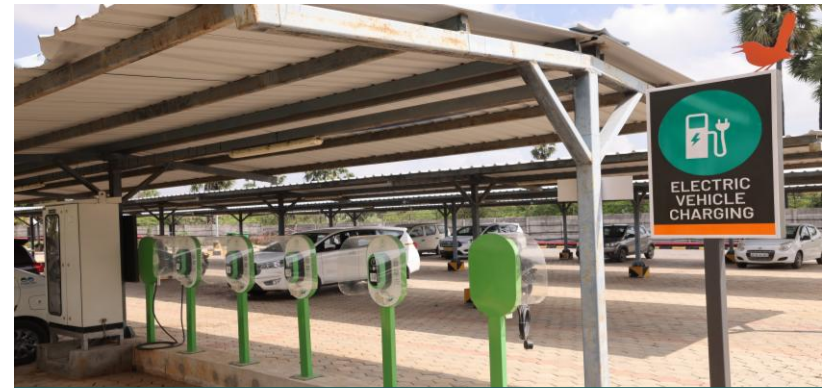
EV charging stations: >150 EV chargers (1 mw capacity)
