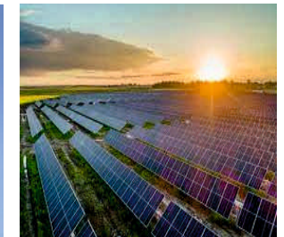
Solar Mounting Structures
