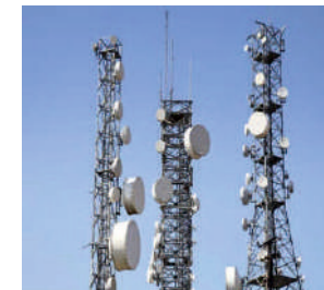
5G Telecom Towers
