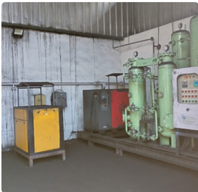
Fig. 6: On-site Nitrogen plant, which is instrumental in kiln cleaning and maintenance
