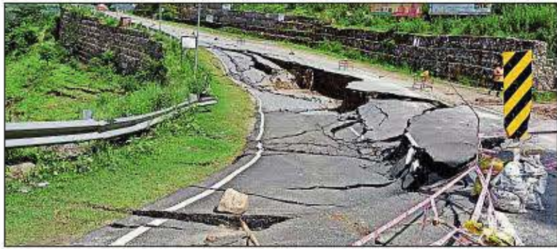
Though temporary repair work is being carried out to make the road safe for vehicles, authorities said that if the situation continues to worsen, traffic will soon have to be diverted
