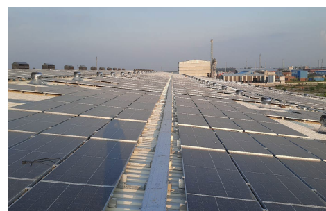
Rooftop Solar Panels at Sandila, Uttar Pradesh
