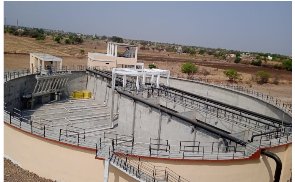
16 MLD Sewage Treatment Plant – Solapur, Maharashtra
