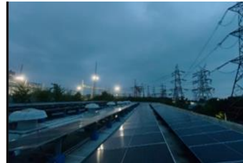
GKEL – 345 kW rooftop solar commissioned
