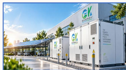
Battery Energy Storage System
