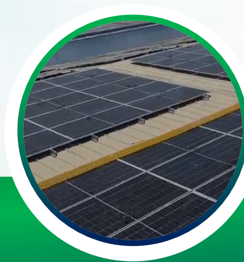
Rooftop Solar System
