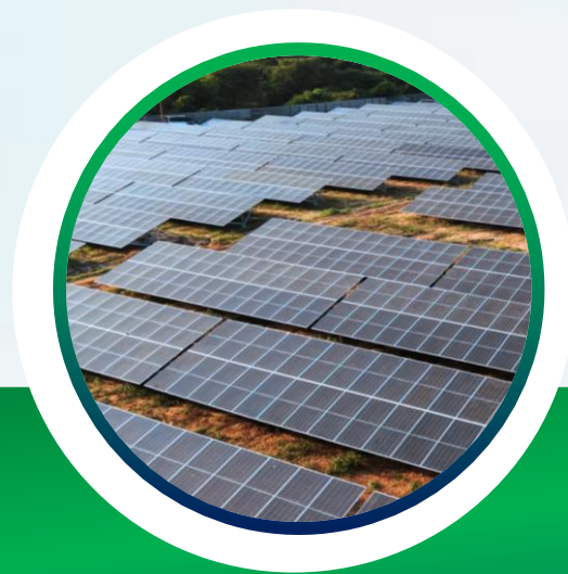
Solar Ground Mounted System
