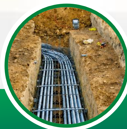
Underground Electric Transmission Lines
