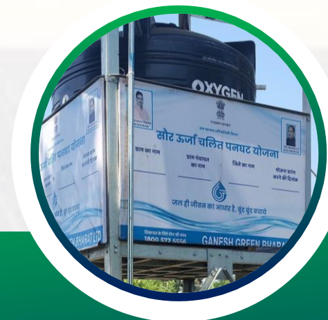
Water Supply System
