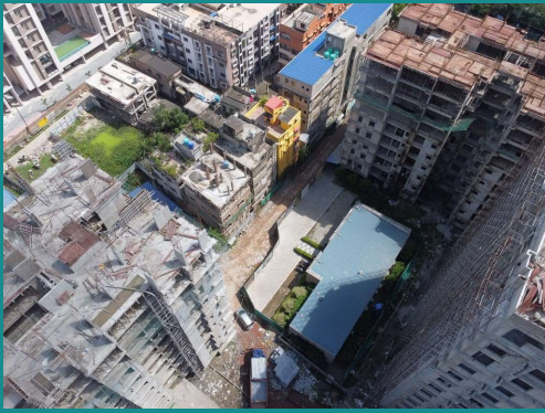
Successfully completed structural work for 5 lakh sq. ft. at the Nucleus Residential Project one month ahead of schedule
