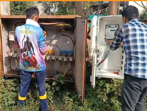
Successfully installed digital smart meters across Maharashtra for Adani Energy: our expertise in large-scale utility Infra
