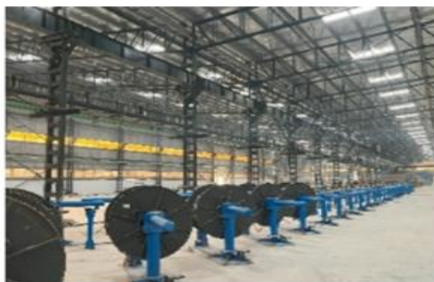
Phase I Furnace Equipments
