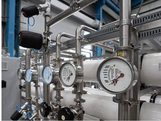
+ Purified Water Generation & Distribution
