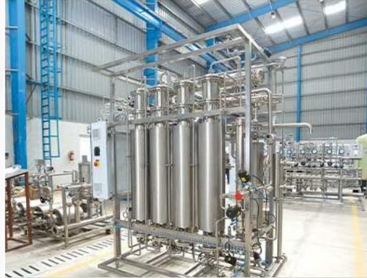
+ Water for Injection (WFI)
